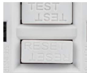
Lockout action blocks the "RESET" button if GFCI protection has been compromised.
